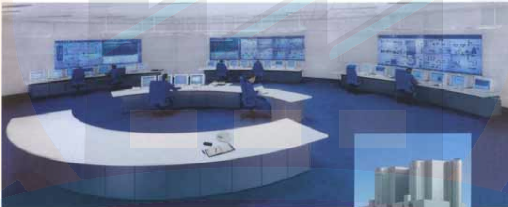
Control room implemented in Schwarze Pumpe, Germany
